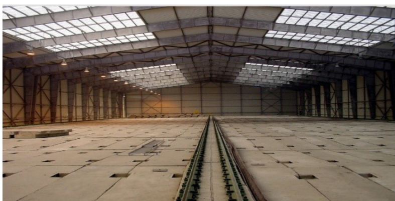
Source: Mochovce Repository, Slovakia. Covered disposal system with chambers protected by concrete panels (courtesy of JAVYS, Slovakia)
